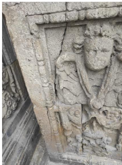
Figure 2. Crack detection (medium) Source: Self-prepared Source: Self-prepared
