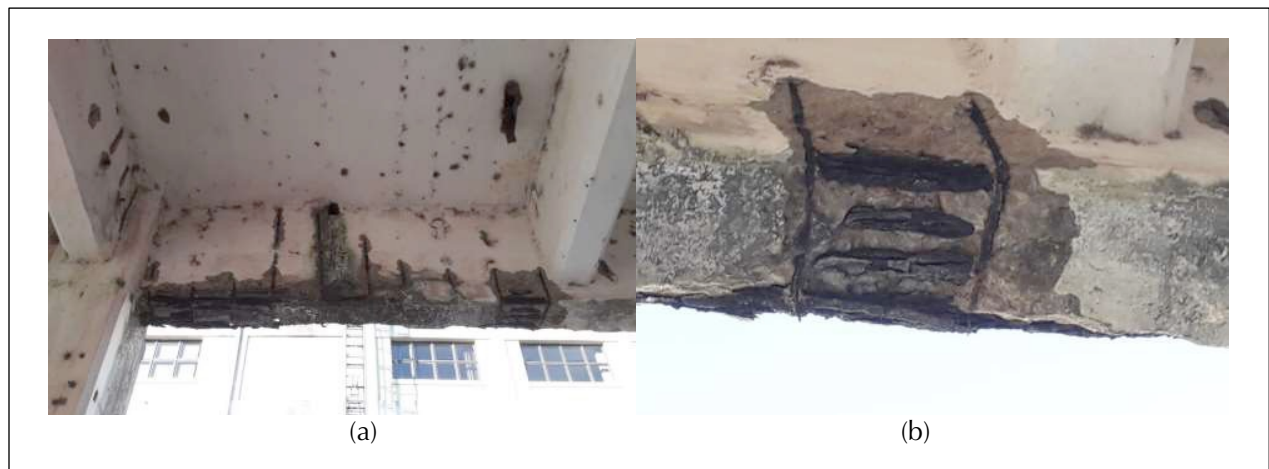
Figure 7. (a) Beam armature exposure and mold stains. (b) Beam with concrete detachment and corrosion and exposure of reinforcements
