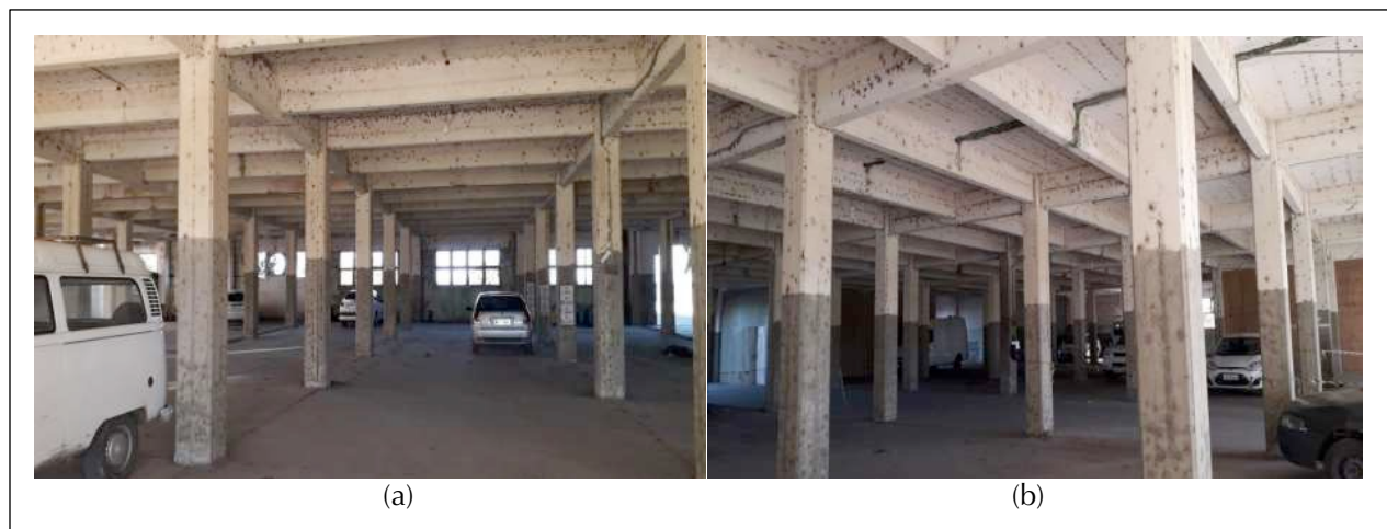
Figure 5. (a) Dirt - North Facade. (b) Dirt - South Facade
