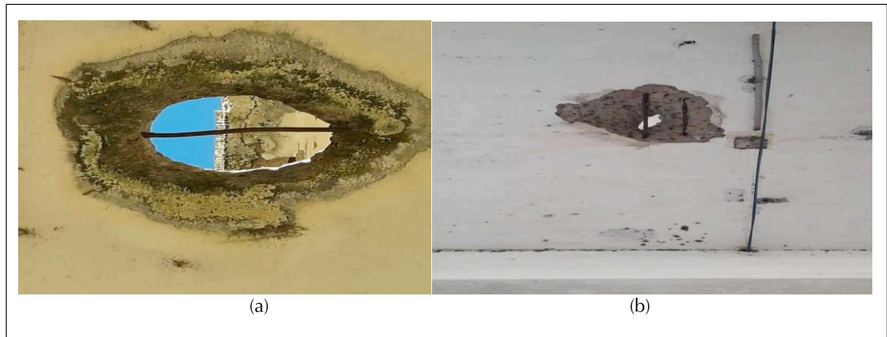
Figure 6. (a) Opening the slab. (b) Slab with peeling and exposed reinforcement
