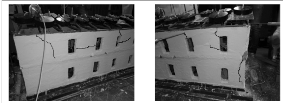
Figure 29. Cracking produced in the back by the seismic activity
