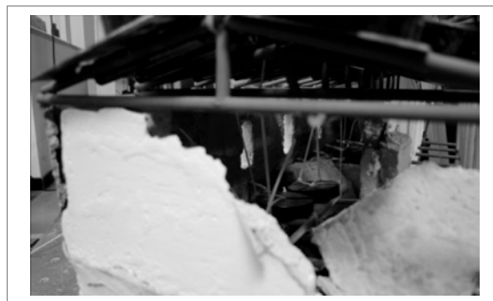
Figure 31. Collapse of the stairways on the second floor
