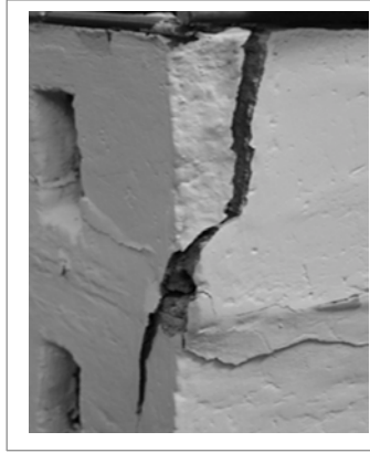
Figure 26. Cracking on the left lateral area after the seismic activity
