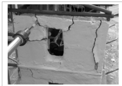
Figure 28. Cracking on the right lateral area after the seismic activity
