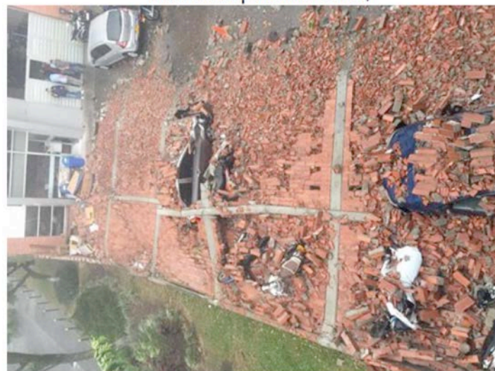
(b) Muro colapsado
