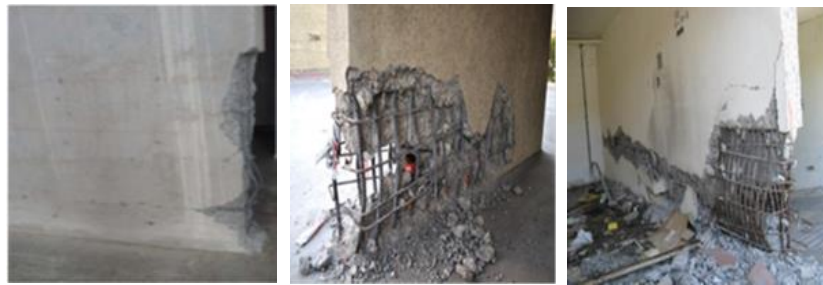
(a) (b) (c) Figure 2b. Examples of reinforced concrete shear walls damaged in earthquakes (Grossi et al., 2011); (Westenenk, B. et al., 2012).
