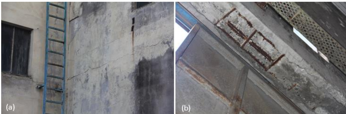
Figure 8. (a) wall cracks, (b) rebar corrosion.
