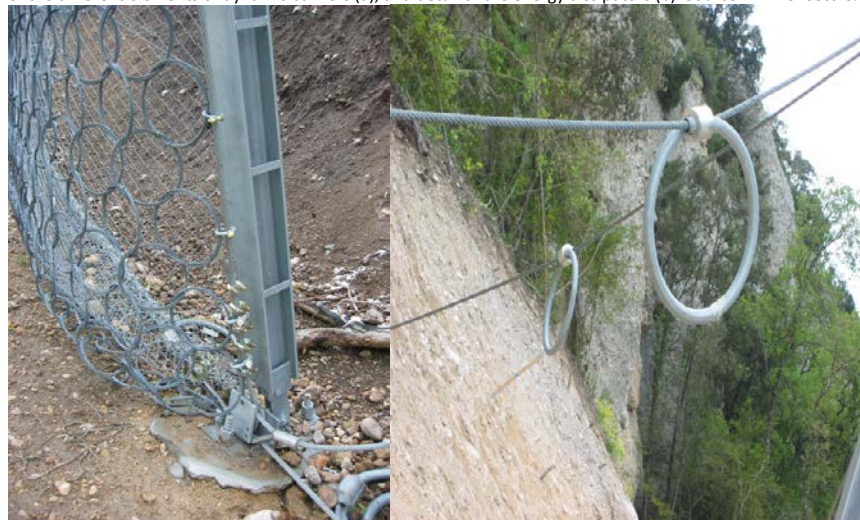
Figure 6. General view of the different elements of dynamic barriers (a), and detail of the energy dissipators (b). Source: R.L. Fonseca & Gonzalez-Gallego, 2007.
