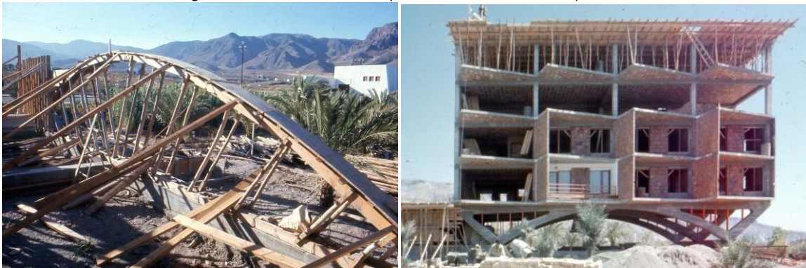
Figure 5a. Arch during construction. 'El Palmeral' apartments. Photo: Cassinello Family archive. Figure 5b. Arch finished. 'El Palmeral' apartments. Photo: Cassinello Family archive.
