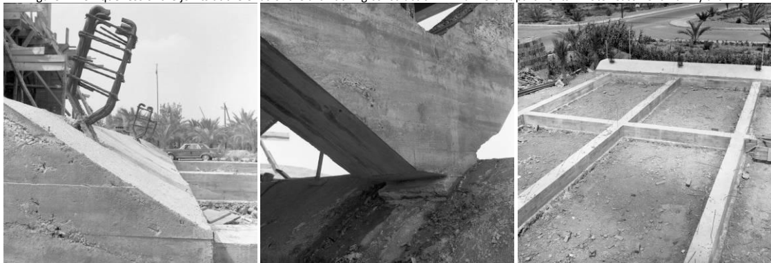
Figure 12. Uniqueness of the joints at the ends of the arch during construction. 'El Palmeral' apartments. Photo: Cassinello Family archive.
