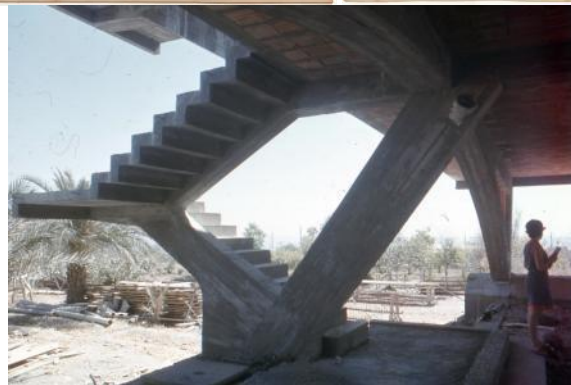
Figure 9a. Stairs during construction, where it is possible to see his daughter Pepa Cassinello on the stringer and staircase finished. 'El Palmeral' apartments. Photo: Cassinello Family archive.
