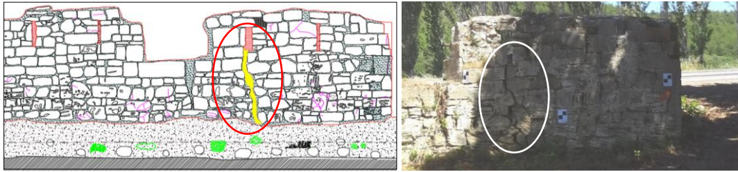
Figure 5. Structural cracks in the south facade walls. Source: Acioğlu (2013).
